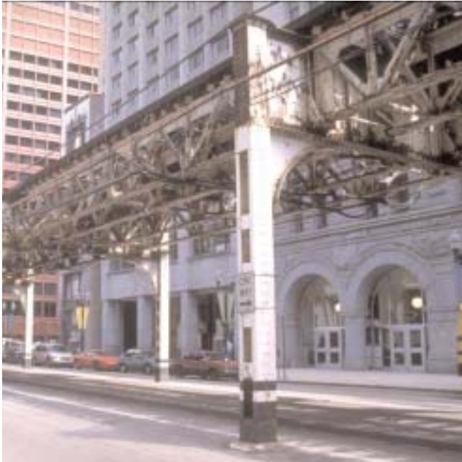
The "L" in deteriorated condition
