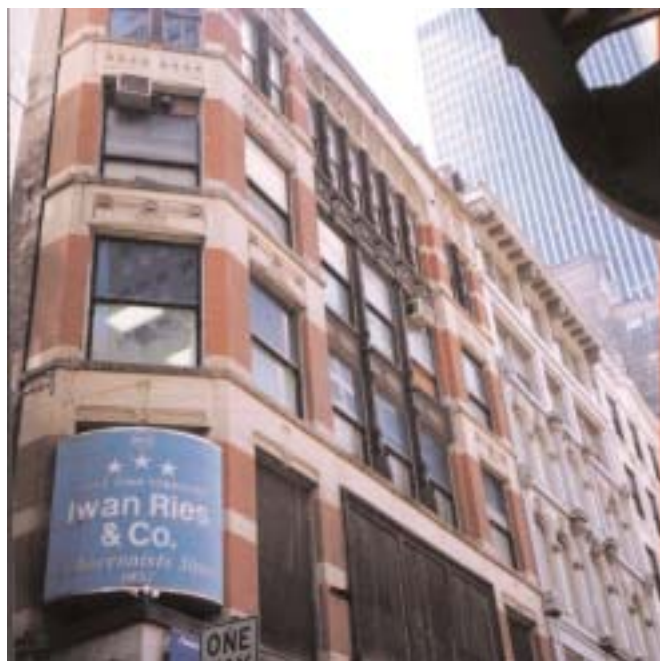
The Iwan Ries Building (Jewelers Building) is the only Adler & Sullivan building other than the Auditorium Building remaining in the Loop, and is in great need of restoration and rehabilitation efforts.
