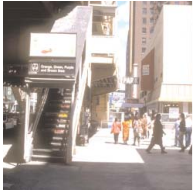
Unattractive and poorly maintained station entrances
